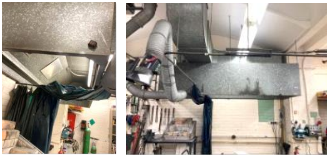
Welding booth (extractor hood ducted)
